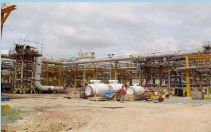
View Spool Tie In G17e/G18e and the Support
